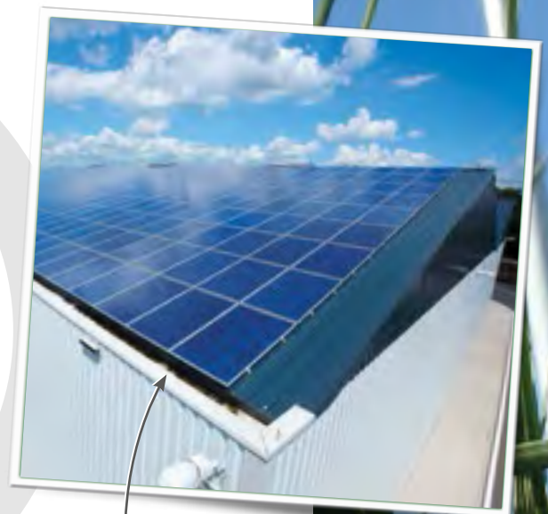
Solar panels provide green energy
